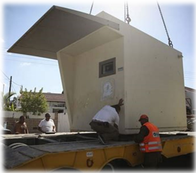
An Israeli mamad prior to installation.
